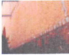
Typical resin flooring.
